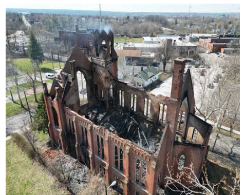
Below: Miles Pentecostal Determine Church after Fire
