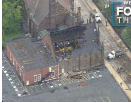
Above: Calvary Church after the storm damage
