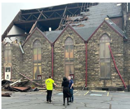
Below: Calvary Presbyterian Tornado Damage, 2022
